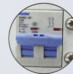
Electrical safety breaker
